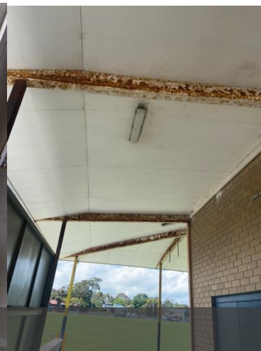
Damage to Ceiling
